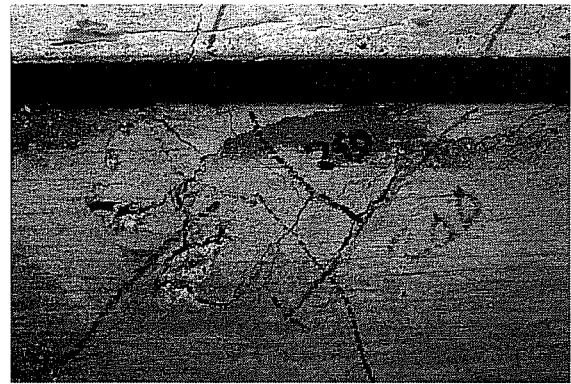
Figure 6.10(b): Close-Up of Spalled Concrete
