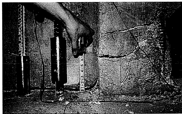
Figure 6.15: Crack Following Splice Failure (West Column)
