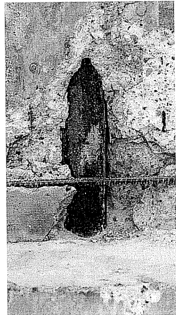
Figure 3.14: Shear Yielding of Pipe (FC-4)
