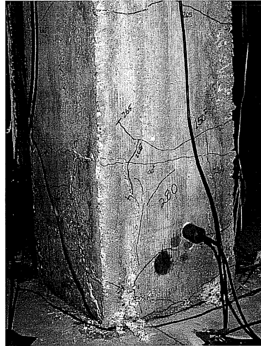
Figure 6.25(b): West Column Splice Failure
