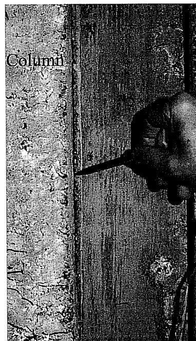
Figure 6.18: Frame Boundary Crack (East Column Shown)
